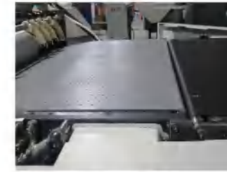
两条分体输送带，降低面纸粘胶风险 Two separate conveyor belts to reduce the risk of sticky glue tissue
